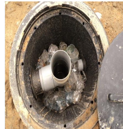
Interior de Biodigestor
