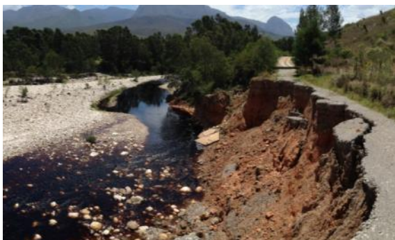
Figure 42 The road wash-away 2014
