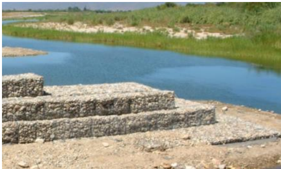
Figure 21 Early Western Cape groyne with vertical edges at the tip that promoted the formation of deep scour holes
